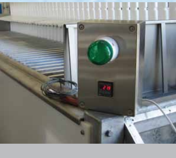
Control box for each freezer.
